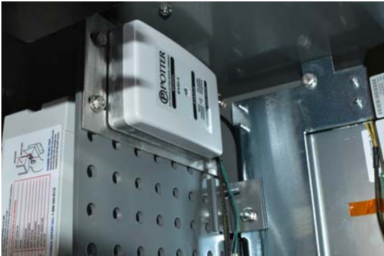
Figure 13. Vandalism Sensor installed on center security wall of the Auto Sentry® CPT
